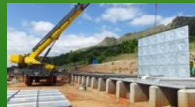
R3 Services at the Zuwini Five-star Hotel Treatment plants installation project with Hydrospec
